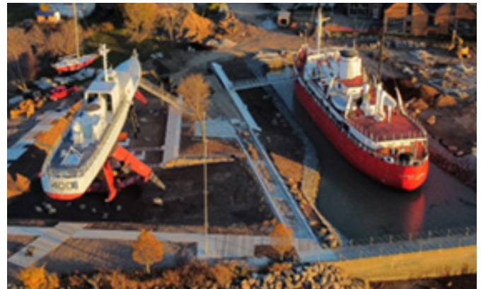
Aerial view of the MMQ riverfront park project, November 8, 2021 - Credit: Pierre Gosselin
